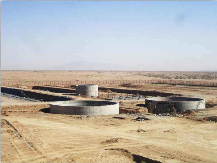
Ardakan Wastewater Treatment Plant
